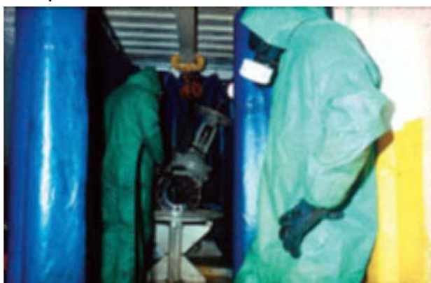
Fig.5. Workers wearing personal protective equipment decontaminating a valve inside an on-site facility.
