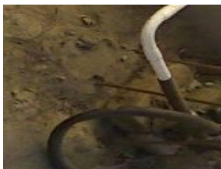
Interval recycling pumping arrangement at the basin Photo (5)
