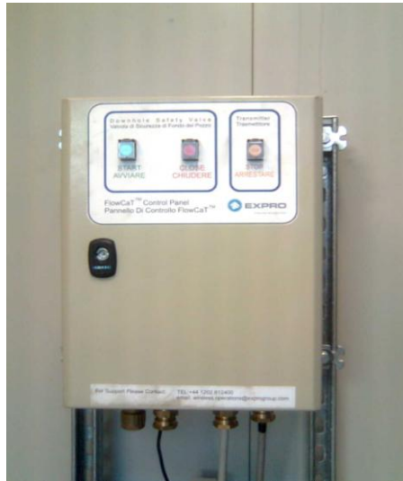
Fig.(3) The control panel.
