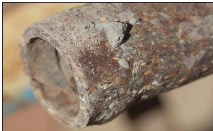
Fig. (5): Corrosion pipe caused by H 2 S [40]
