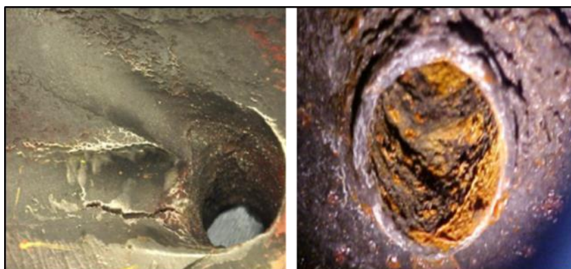
Fig. (6): Corrosion caused by \text{NH}_4\text{HS} [46]
