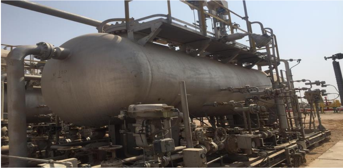
Fig. (1): 1 st stage test separator (20-V-100) at Hammar Mishrif station, Zubair oil field
